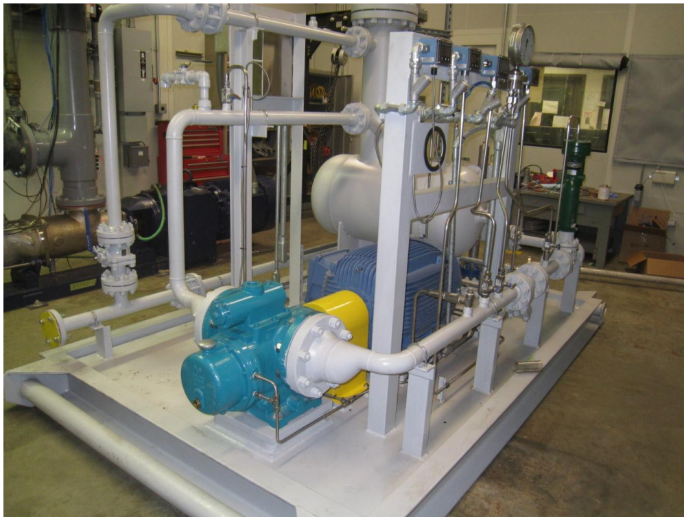
Figure 5.3: Leistritz pump assembly
