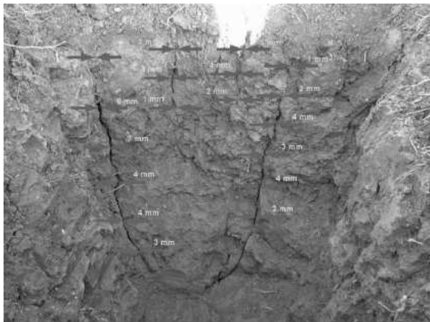
Figure 5.8. Picture showing cracks of different depth and aperture (after Dyer et al., 2009)
