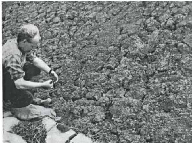
Figure 5.5. Picture depicting cracks on the surface of a flood embankment (after Cooling and Marsland, 1953)
