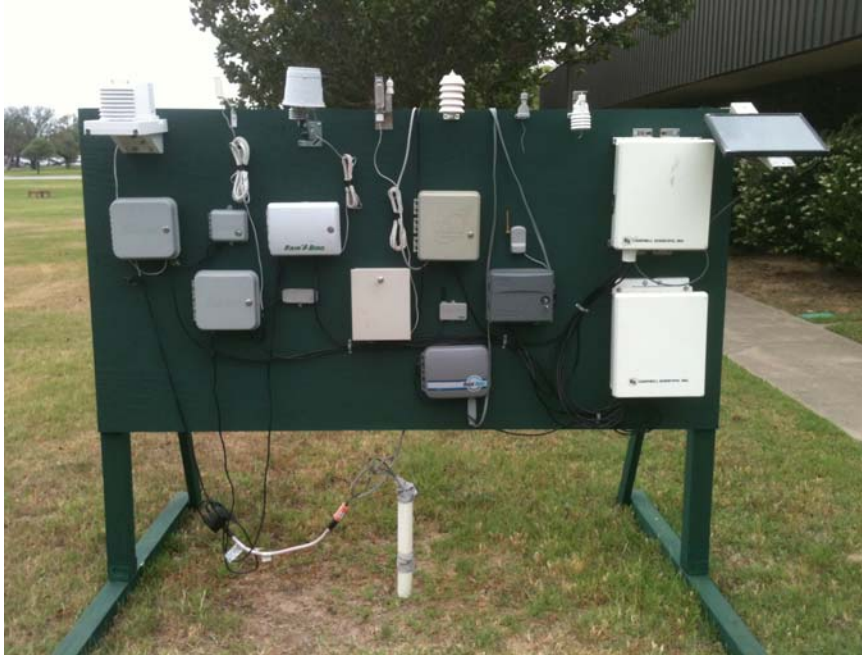
Figure A-4. Outdoor Tested Controllers
