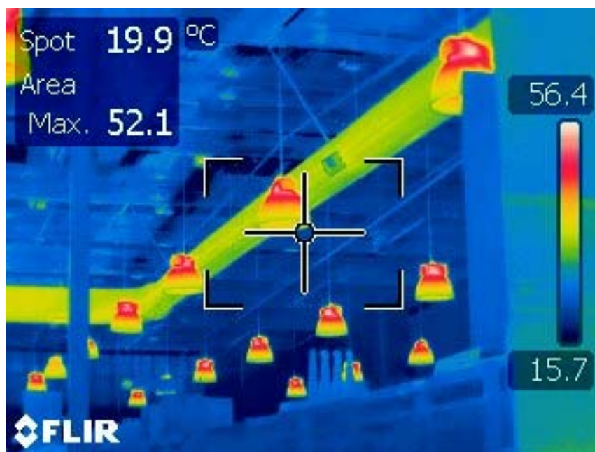
Fig. 12. The AC system supplying warm air to heat the building
