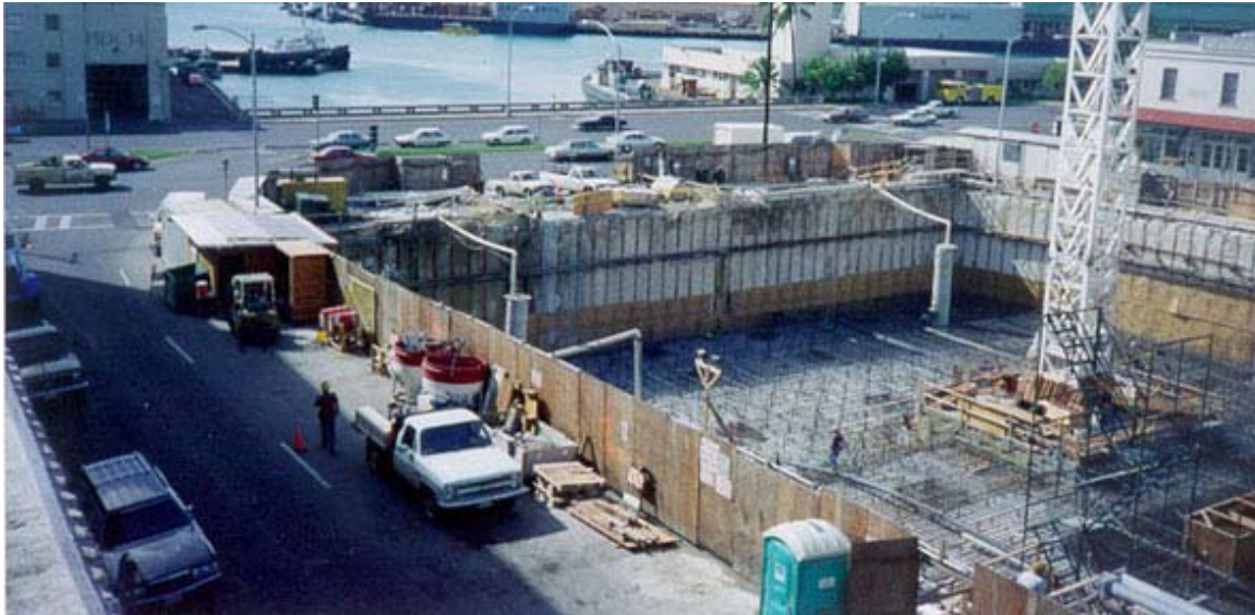
Figure 4 – 5. Marin Tower, Honolulu, HI Project Site (Picture from Schnabel Foundation Company, www.schnabel.com )
