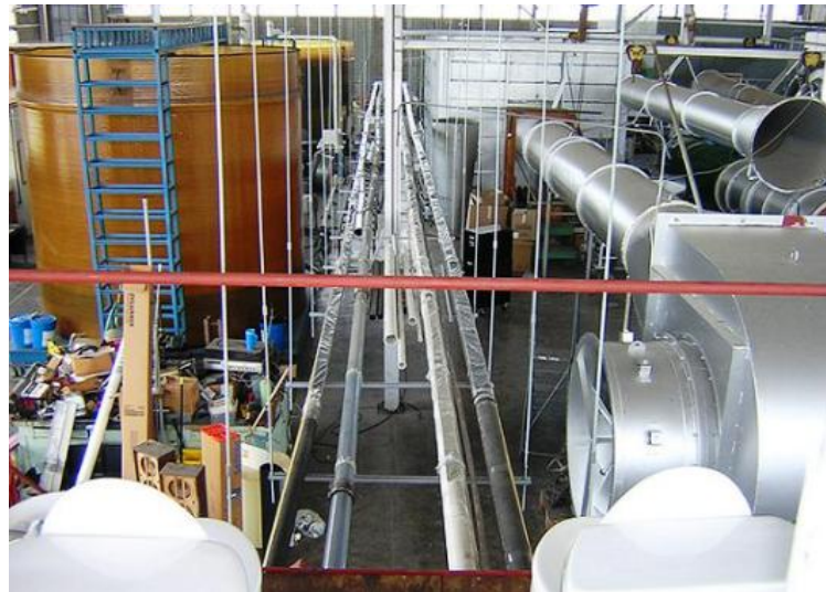
Figure 3: Pipes Viewed from Platform
