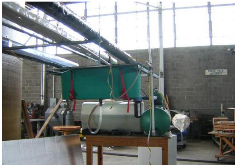
Figure 4: Media Capture Tank, Reservoir, and Pump
