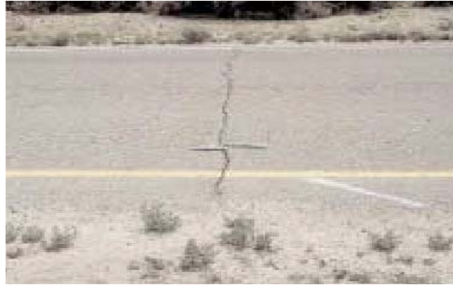
FIG. 2.4. Transverse Cracking (LTPP Distress Identification Manual, FHWA 2003)
