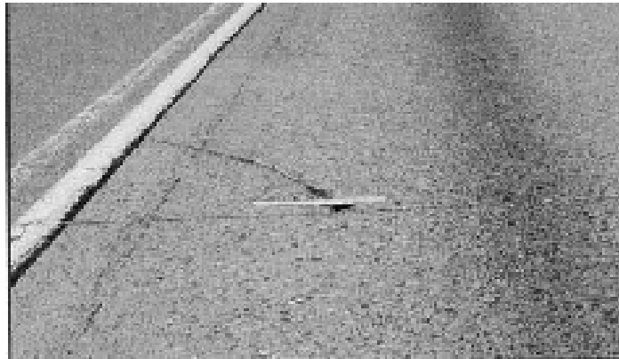
FIG. 2.8. Corner Break (TM 5-826-6/AFR 93-5, USACE 1989)
