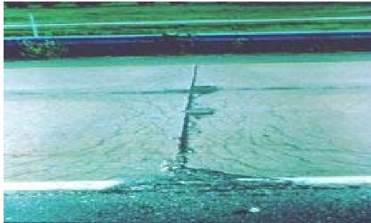
FIG. 2.2. High Severity “D” Cracking (FHWA, 2002)
