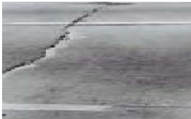
FIG. 2.5. Faulting Distress (LTPP Distress Identification Manual, FHWA 2003)
