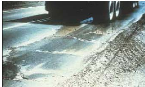
FIG. 2.10. Pumping Distress (LTPP Distress Identification Manual, FHWA 2003)
