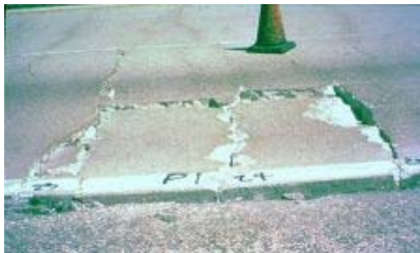
FIG. 2.6. High Severity Punchout (FHWA, 2002)
