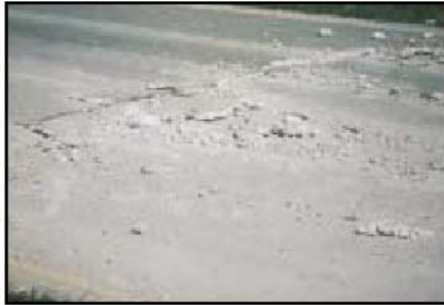
FIG. 2.11. Blowup Distress (LTPP Distress Identification Manual, FHWA 2003)
