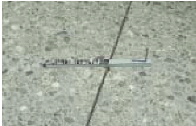
FIG. 2.3. Joint Seal Damage (LTPP Distress Identification Manual, FHWA 2003)
