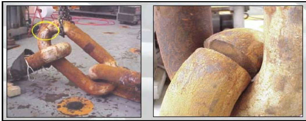
Fig. 2.15: Fatigued sections of a mooring chain Source: TEKNA Conference on DP and Mooring of Floating Offshore Units [7]
