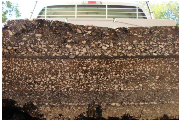
Figure 1.1. Rutting in the asphalt pavements as a result of evolution of the viscoplastic strain. This section is related to US 287 highway in Wichita Falls near Dallas Fort Worth.
