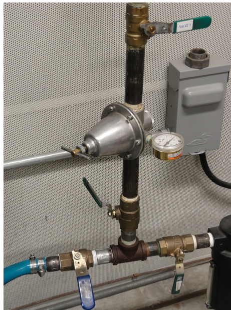
Fig. 69.: Butterfly and throttle valves for calibration facility
