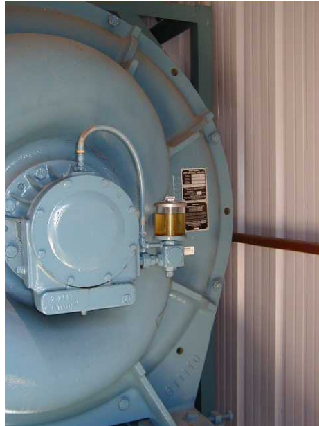
Fig. 87.: Oil level indicator for compressor
