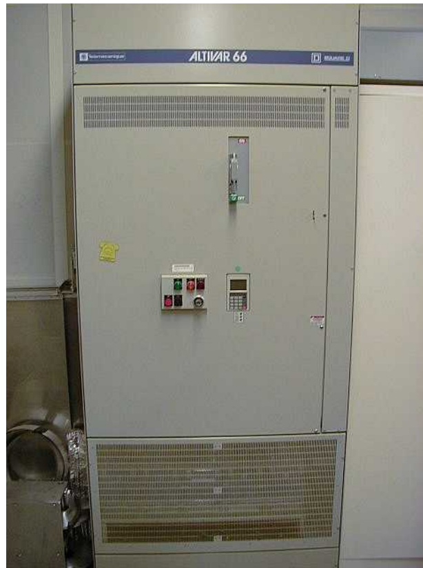
Fig. 91.: Variable frequency controller for compressor
