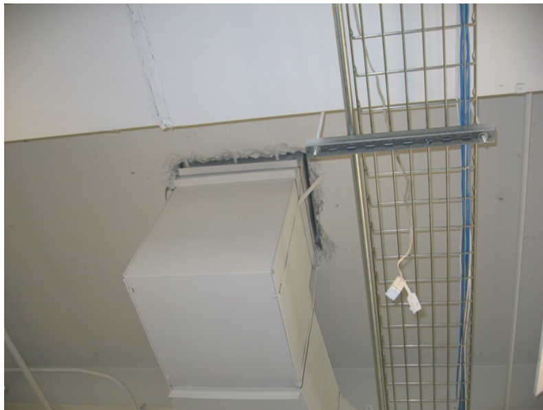
Figure 6.13 Potential Leakage Points - Where Ducts Penetrate the Third Floor Ceiling
