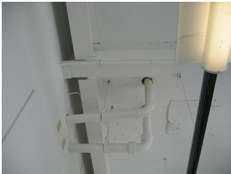
Figure 6.15 Potential Leakage Points-Drain Pipe Penetrates the Third Floor Ceiling
