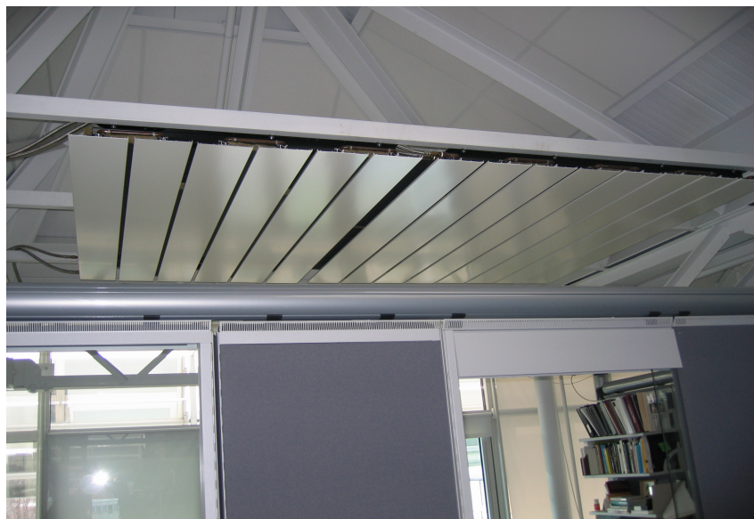
Figure 1.2 The Overhead Radiant Panels
