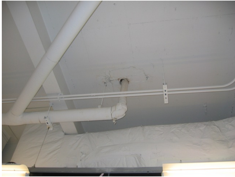
Figure 6.14 Potential Leakage Points-Where Pipeline Penetrates the Third Floor
