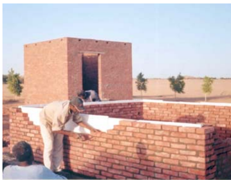
Figure 2. Photo of room built from double layer of hollow clay brick and thermal insulation in between
