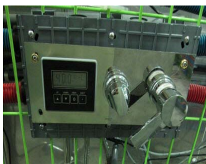
Figure 4 Temperature control box
