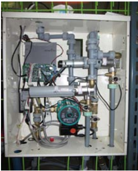
Figure 6 Thermal valve box
