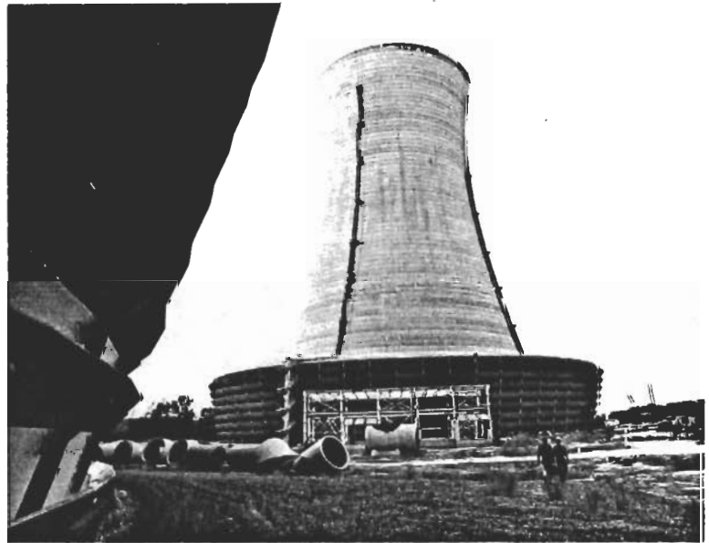
Figure 8. The size of the cooling tower is relative. Energy conservation techniques are the same for large or small counter-flow or crossflow configurations.
