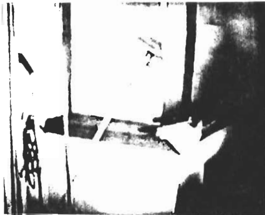
Air handler unit sitting on return plenum located in garage.
