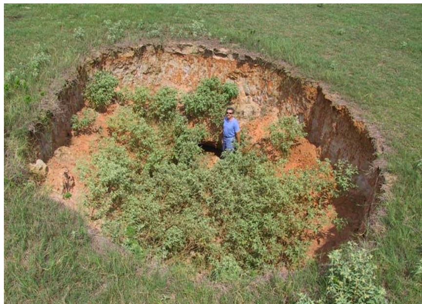
Fig. 6. Surficial subsidence features (sinkhole) at Malakoff. Mr. William Reimer in (high priority) Sinkhole S-4 at Malakoff, Texas (Source: RRC Texas)
