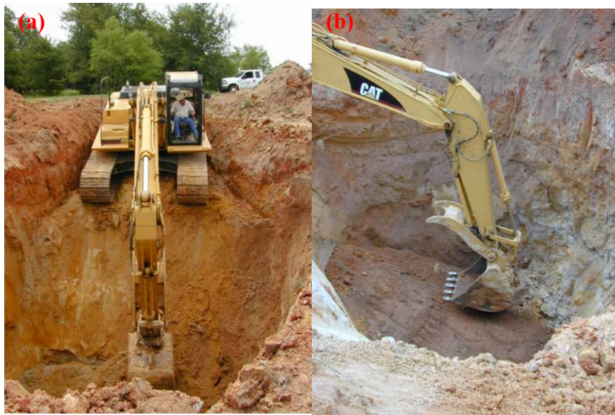
Fig. 32. Reclamation process at Malakoff (July 2003). (a) Backhoe used to dig and remove soil from a sinkhole, (b) Backhoe thumping the ground to compact the soil while filling the sinkhole
