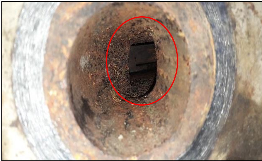
View from Discharge Nozzle: Impeller not centered in the opening
