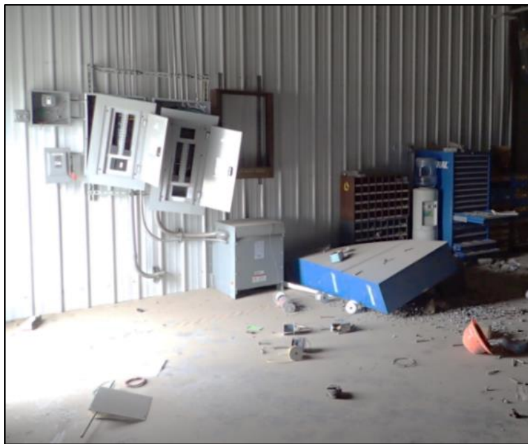
Figure 3. Wall mounted Non-Structural Building Debris
