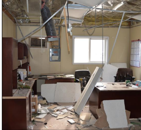
(b) Post-blast event overhead debris
