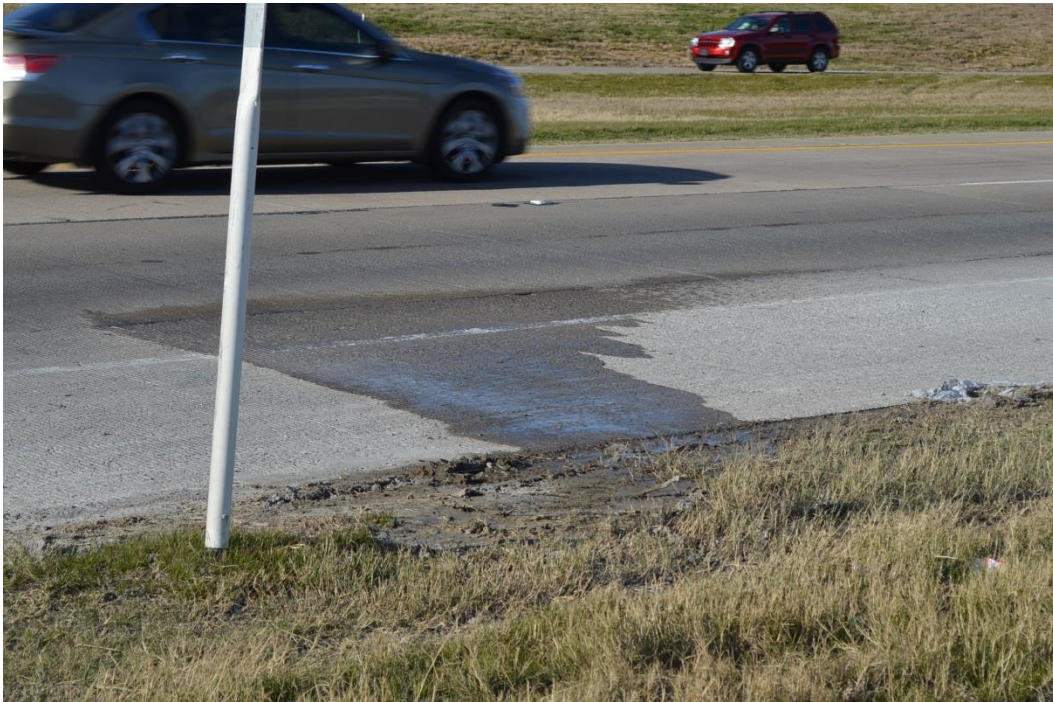
Fig. 1. Water pumping through a pavement structure due to inadequate surface drainage and pavement distress
