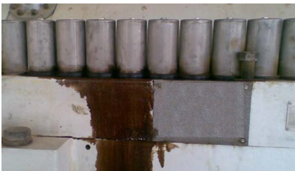
Figure 11. Observed Leakage during operation on site.
