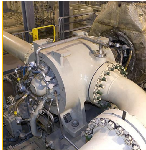
Figure 1. Compressor model at a site installation and driven by a gas turbine engine
