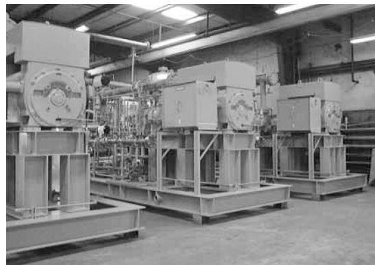
Figure 3. Motor-Driven Fuel Gas Booster.
