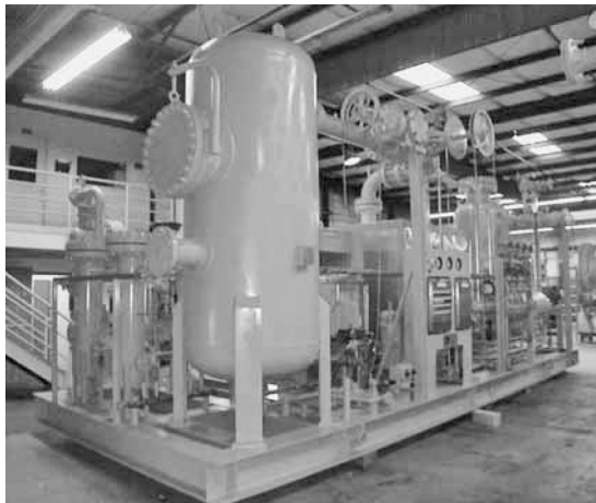
Figure 5. Motor-Driven Refinery Gas and Natural Gas Compressor.
