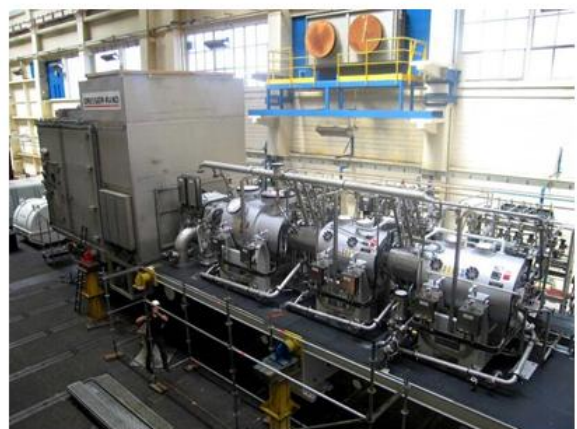
Figure 5. A three case gas reinjection compressor train driven by an aero-derivation gas turbine destined for installation on an FPSO.
