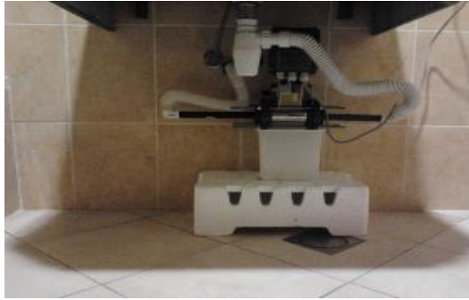
Washbasin water collection
