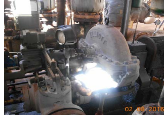
Unit 1C – FBS Upgrade
