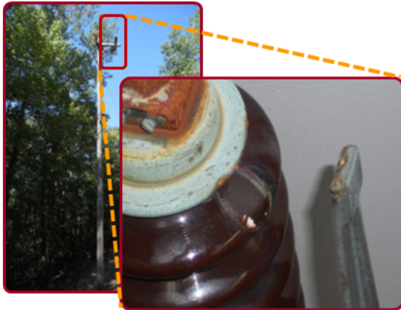
Figure 7.16: Picture of failing arrester
