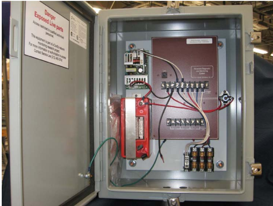
Figure 15: NEMA enclosure with DCD installed
