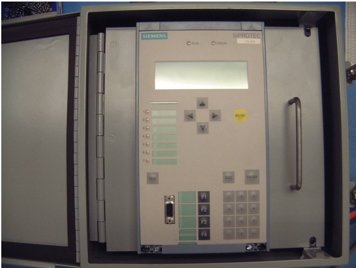
Figure 7: Installed enclosure containing Siemens 7SJ64 relay
