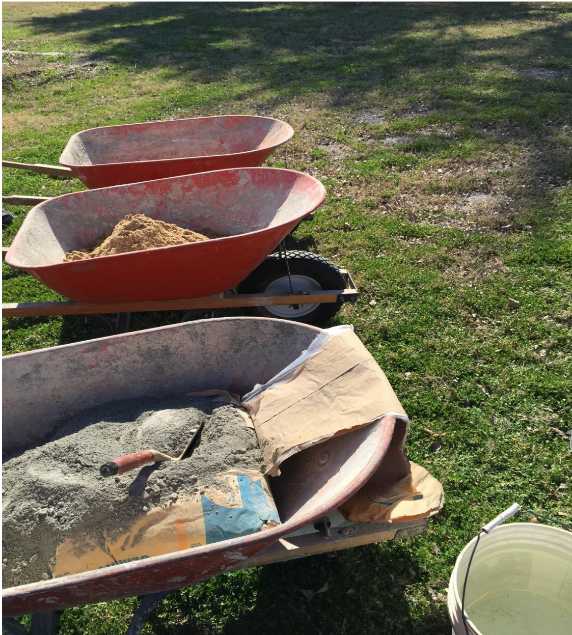
Figure 18: Lime, sand and cement gathered together and measured before being added to the concrete mixer
