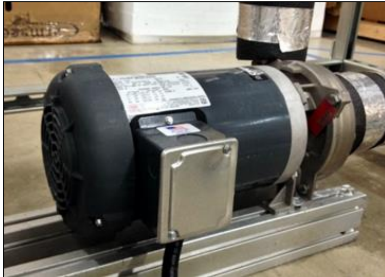
Figure 13. Stainless-steel centrifugal pump
