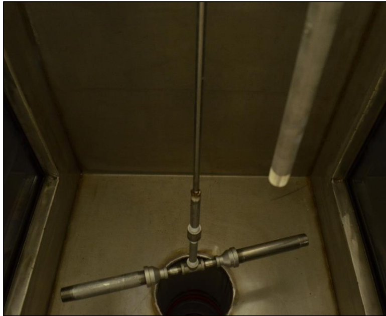
Figure 11. Mixing propeller inside of tank
