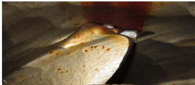
Figure 37. Close-up view of the middle right image in Figure 35. A white cloth was placed behind the diffuser to clearly show two through thickness holes developed at the diffuser vane leading edge and sidewall intersection point.
