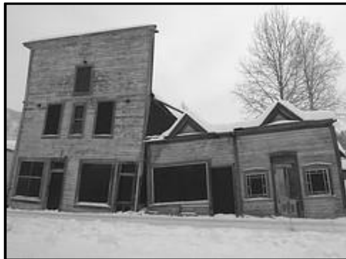
Figure 1.5 Large settlement observed in residential homes in Dawson City, Yukon (Varani, 2000)
