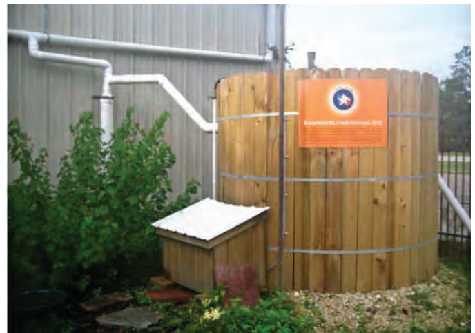
Rainwater harvesting system
