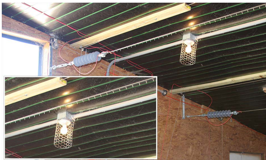
Figure 1. Corona lines running from power source.
