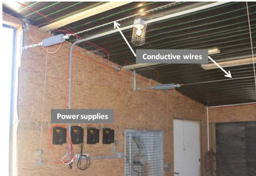
Figure 2. The ionization units hanging from the ceiling of the broiler treatment house and connected to the power supplies.
