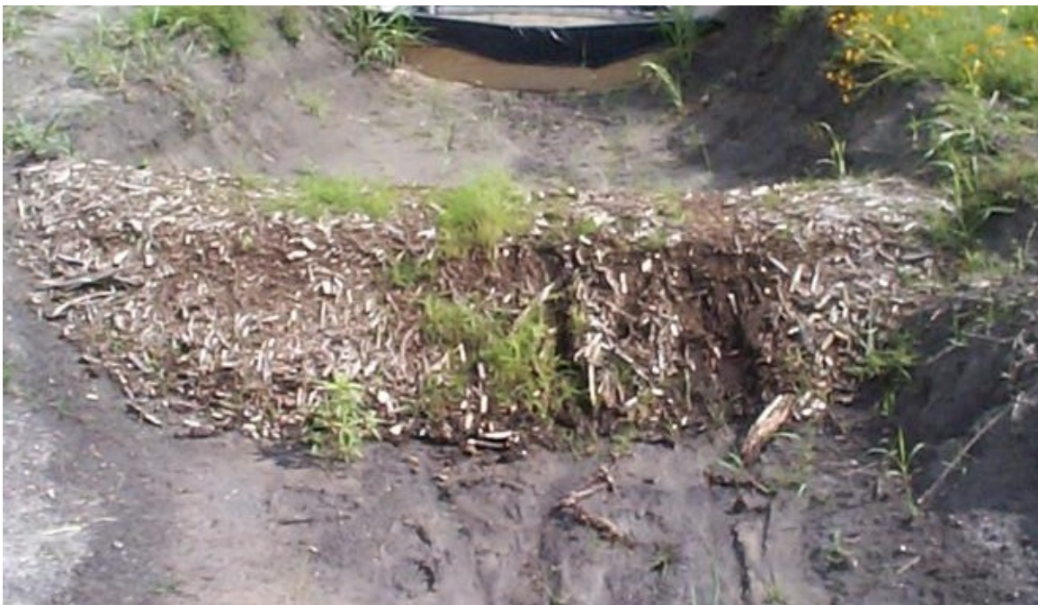
Figure 5.39 Composted bio-solids berm showing minor damages to the leading face.
