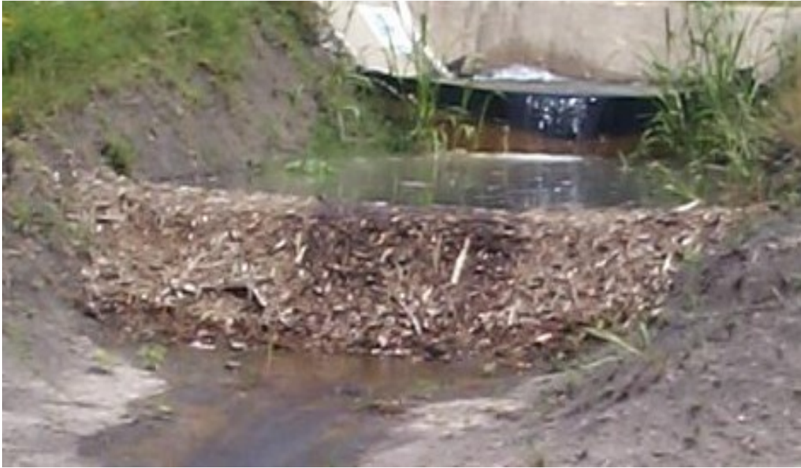
Figure 5.41 Yard waste compost berm showing no damages to the leading face.
