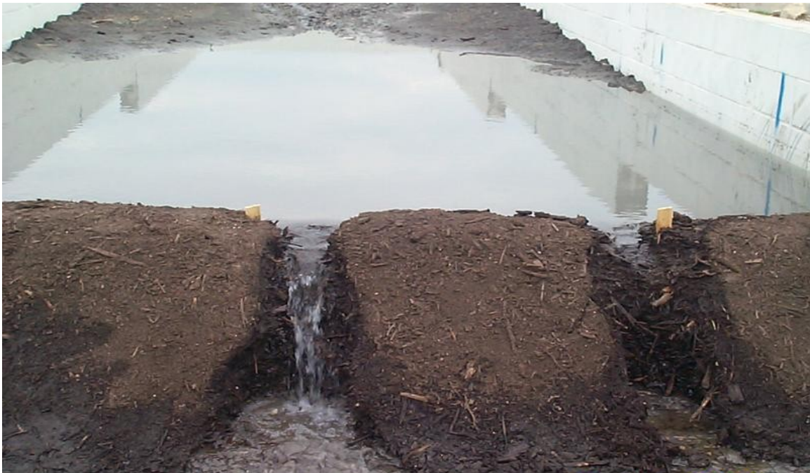
Figure 5.5 Failure around the stakes when the berm was anchored.
