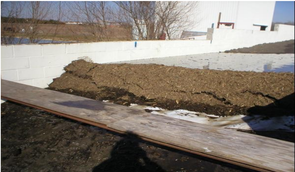
Figure 5.4 Displacement causing stresses leading to failure of the berm.
