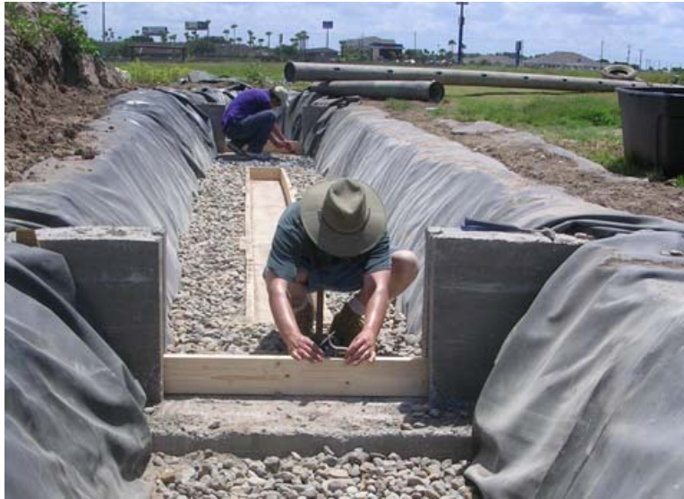
Fig. 3.3 Setting and caulking stop logs for control structures in field channel. Note central slot for placement of trays holding vegetation
