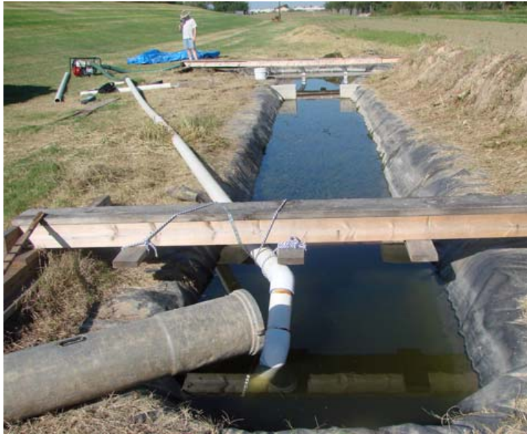
Fig. 3.4. Field channel with pump and piping system in place. Note hydrilla growing in the test section
