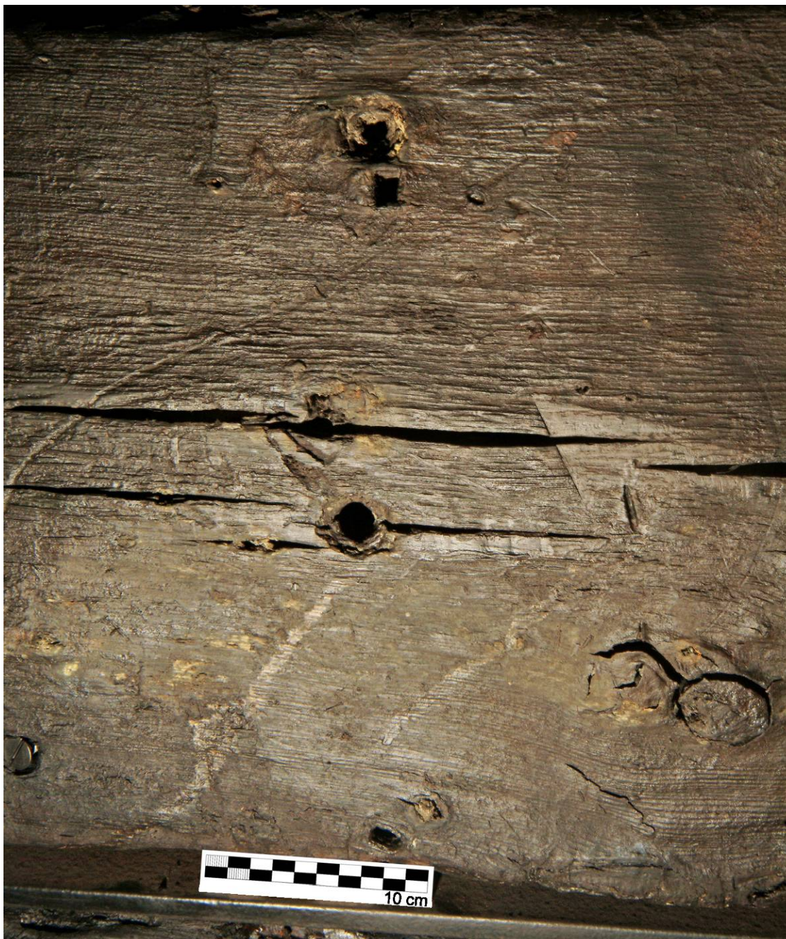
Fig. IV.23 Nail holes on exterior of inner layer of hull planking directly forward of transom. Nail head impressions with nail holes are from fasteners that fixed the inner layer to frames, whereas each nail hole next to them, are from nails that fastened the outer layer of planking to inner layer, Batavia shipwreck, BAT 6389. Photograph: Patrick Baker, Western Australian Museum.
