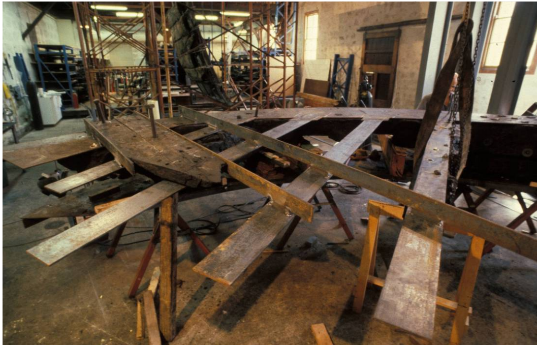
Fig. III.26 Constructing the steel support for the transom planking on the backing plate of the fashion piece and transom beams, Shipwreck Galleries of the Western Australian Museum, Fremantle. Photograph: Brian Richards, Western Australian Museum (BT-T-0239).
