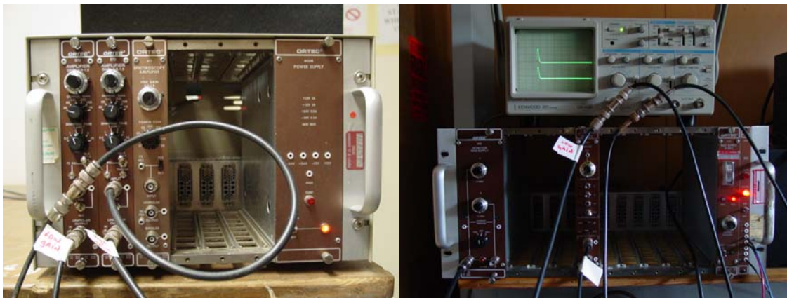
Figure 2.16. Detector's NIM bins. Left: Power Supply and amplifiers. Right: detector Bias Supply and Pulser.
