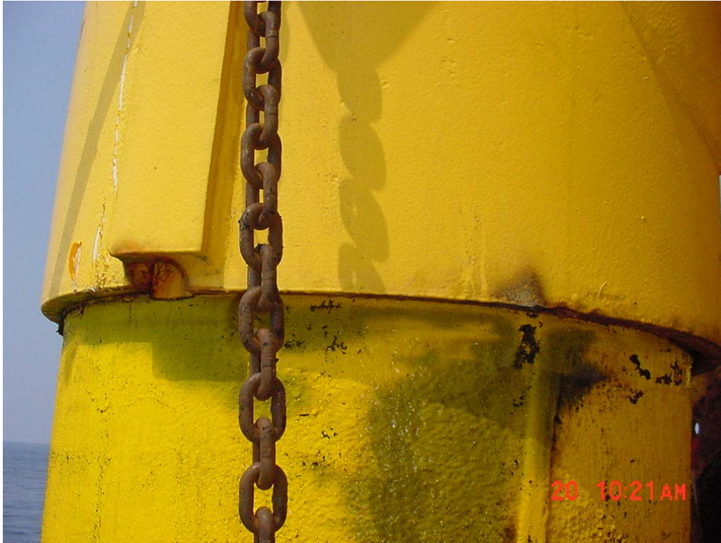
Figure 2 – A conventional riser repair involving a welded steel clamp
