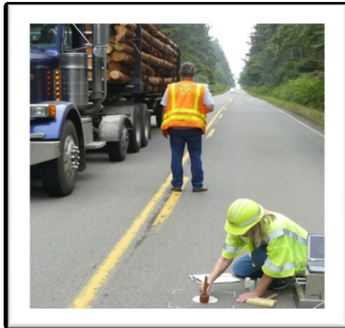
FIGURE 4 Sand patch testing for pre-existing pavement macrotexture before chip sealing in Washington state: spreading glass beads into a circle.
