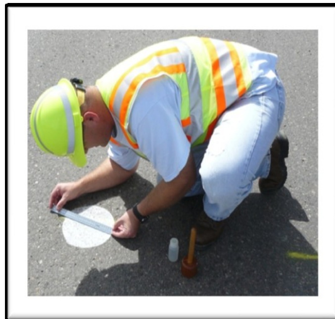
FIGURE 5 Sand patch testing for pre-existing pavement macrotexture before chip sealing in Utah: measuring diameters of the circle of glass beads.
