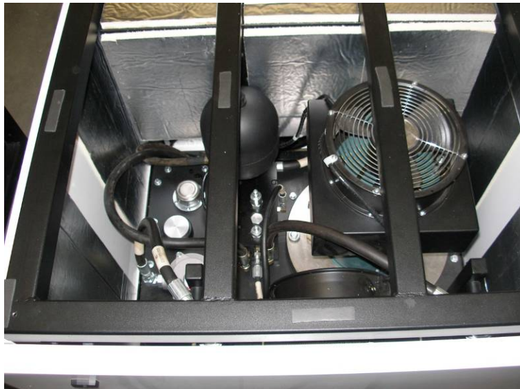
Fig.3.8. Hydraulic power supply.
