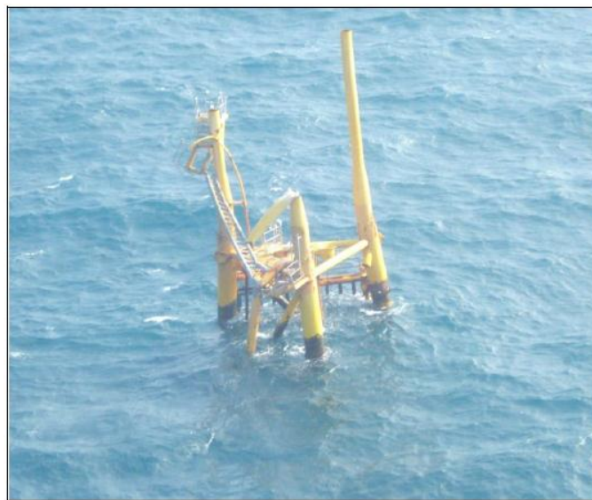
Fig. 7 —Destroyed platform in the Eugene Island Area from Gustav and Ike in 2008 (BOEMRE, 2010).
