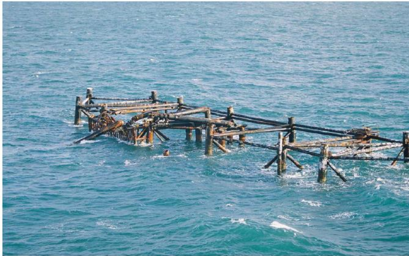
Fig. 5 –Destroyed platform in the South Timbalier region after Katrina and Rita in 2005 (BOEMRE, 2007).
