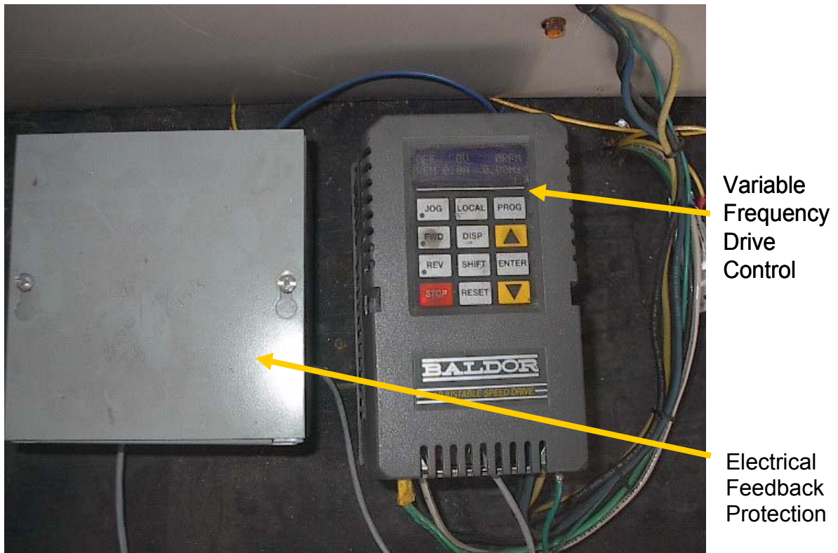
Figure 21. Variable Frequency Drive
