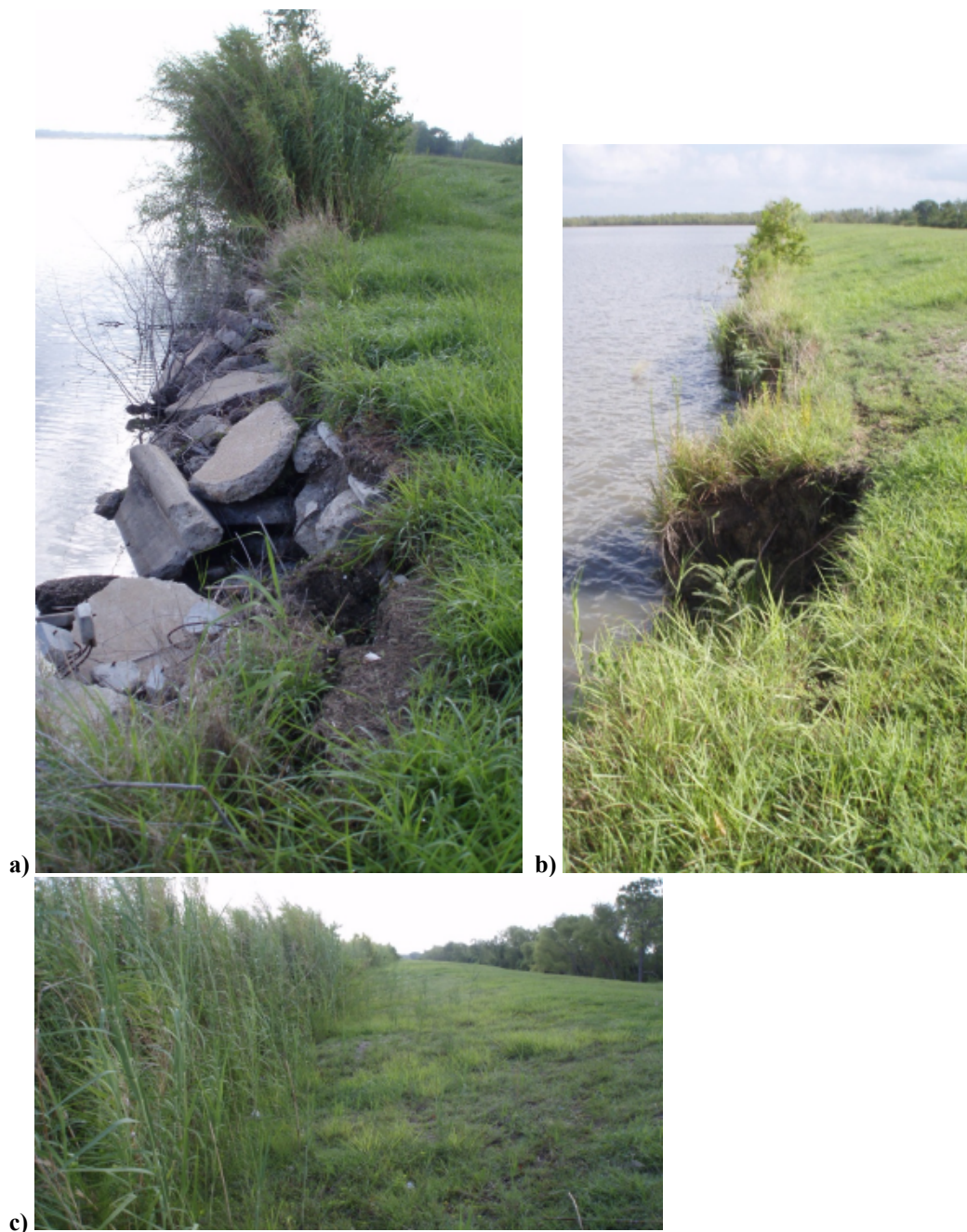
Figure 5.7. Pictures of Highlands Reservoir embankment levee. This includes (a) picture showing concrete rubble riprap and erosion, (b) unprotected embankment section with significant wave erosion, and (c) tall, dense reed growth that prevents inspection and provides burrowing habitat for animals. Images produced with permission from FNI and SJRA.
