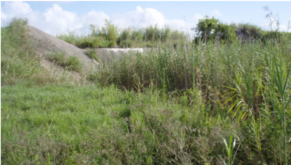
Figure 5.8 Picture of existing emergency spillway in disrepair. Produced with permission from FNI.
