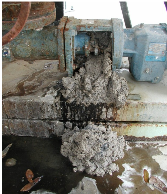
Figure 2-21. Picture of biomass leaking out around pump packing.
