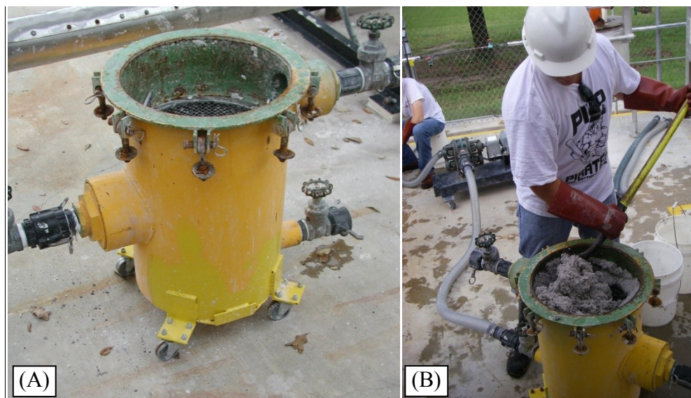
Figure 2-14. Pictures of (A) empty oilfield-style filter tank, and (B) fermented office paper and chicken manure being filtered in filter tank with gear pump used to pull vacuum via 2-inch transfer hose.
