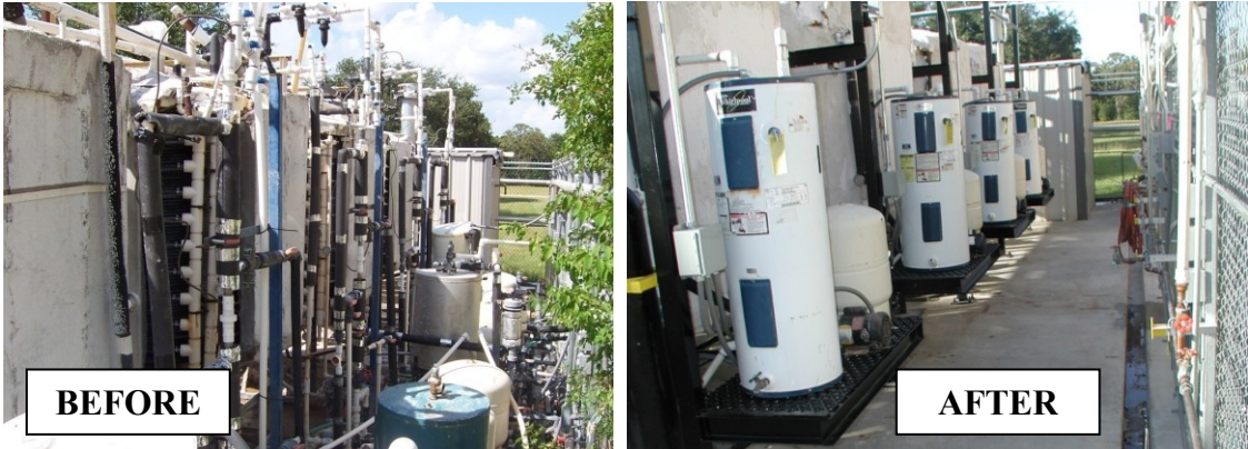
Figure 2-9. Pictures of water heaters and plumbing behind fermentors before and after renovation.
