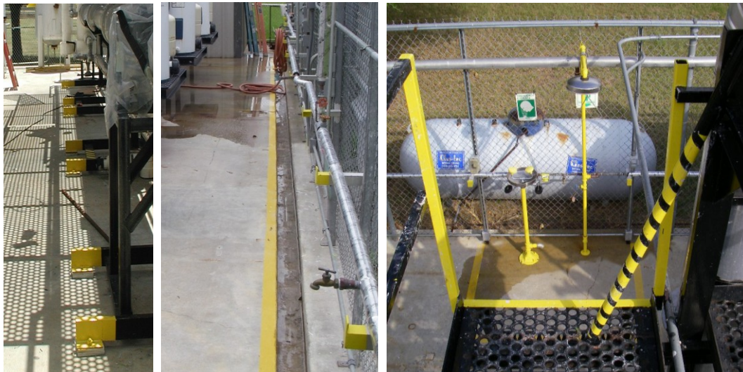
Figure 2-3. Pictures of places where safety yellow paint was used to identify potential safety hazards. Safety shower and eye wash station are shown in right-most picture.
