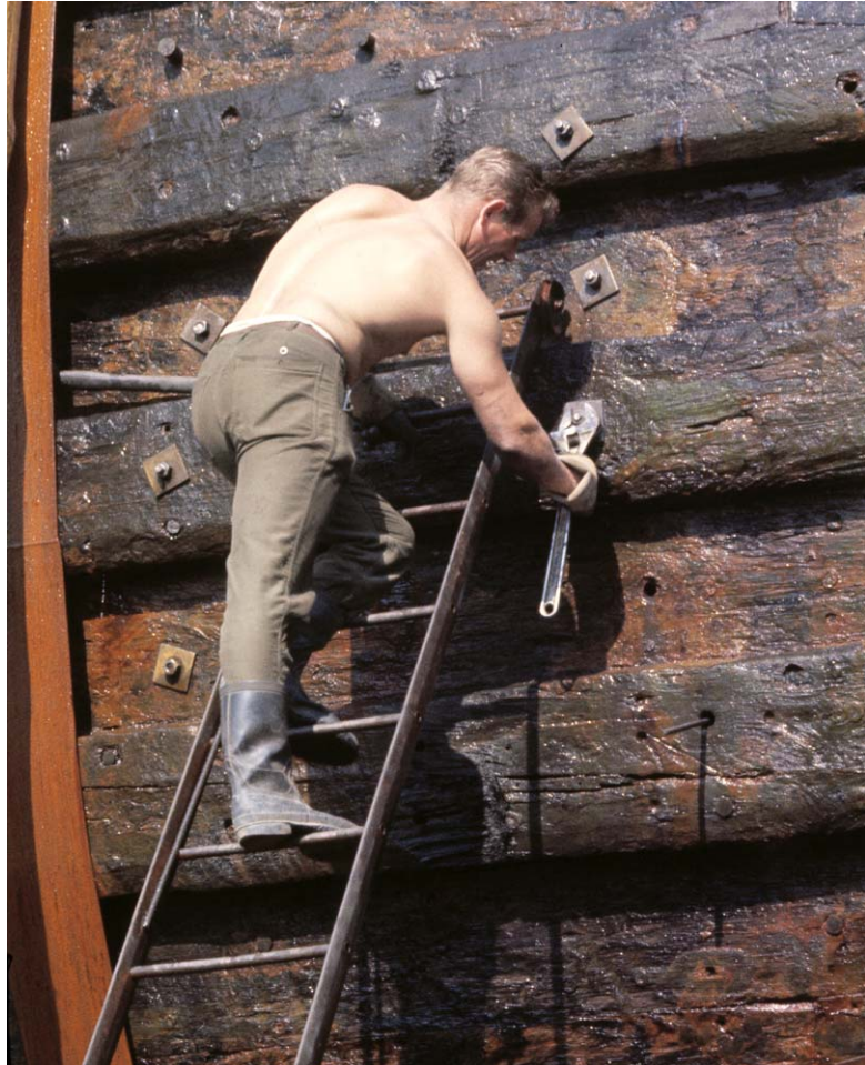
Figure 10. Replacing the rusted away original bolts. New epoxy coated galvanized mild steel bolts were inserted into the empty original bolt holes (Courtesy Archives, the Swedish National Maritime Museums).
