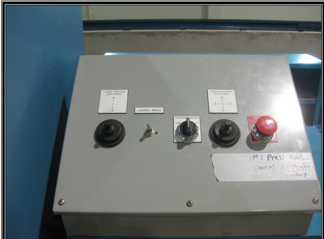
Figure 20. Control panel and knobs for driving the dredge carriage electronically and remotely.
