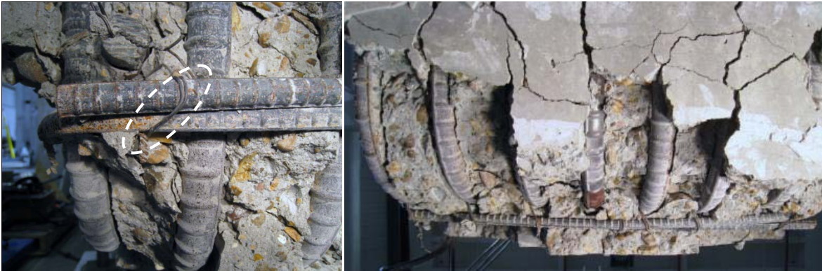
(c) Debonding of transverse U-bars
