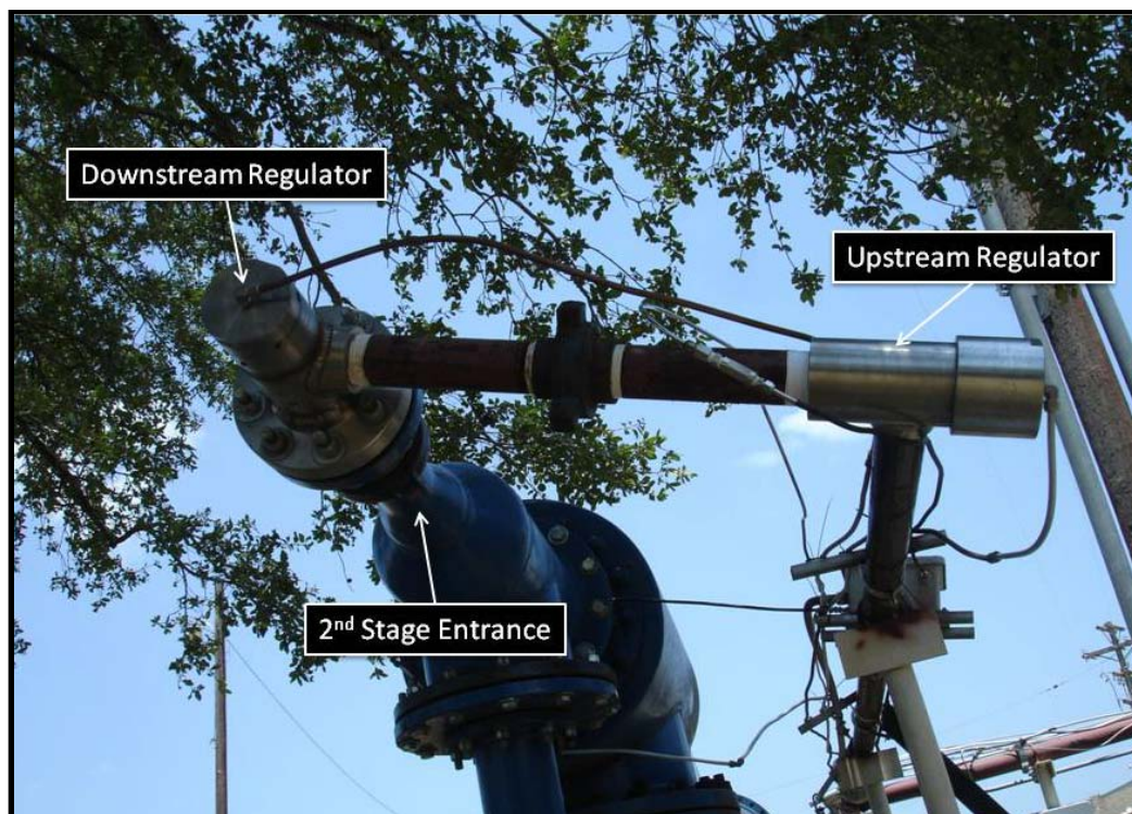
Figure F-8: Ejector 2 nd Stage Air Supply Line
