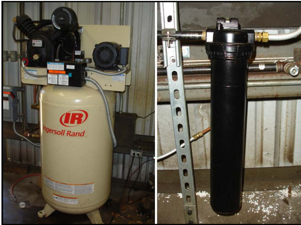
Figure 22: Actuator Air Supply Compressor and Dryer
