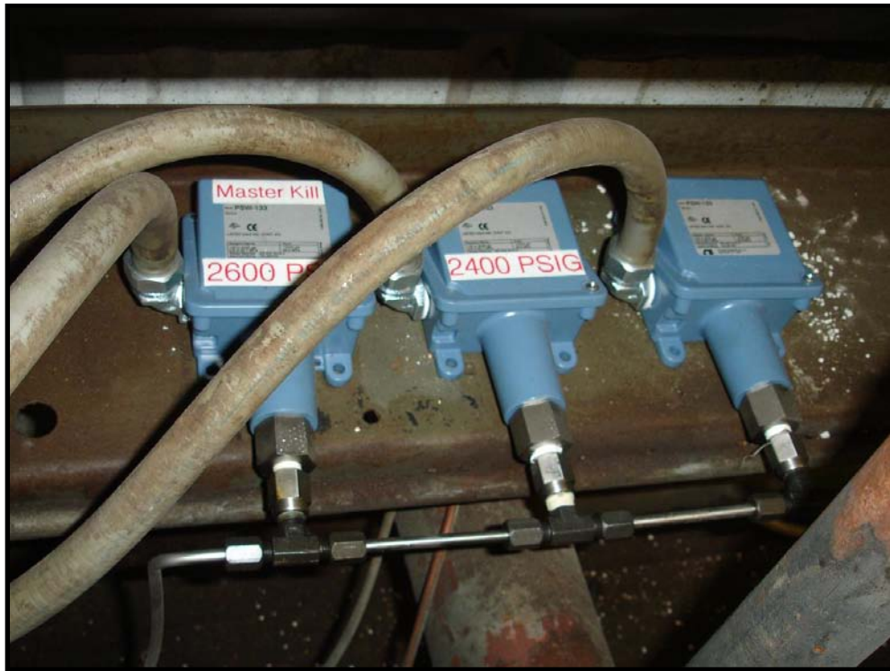
Figure 8: Compressor Pressure Switches
