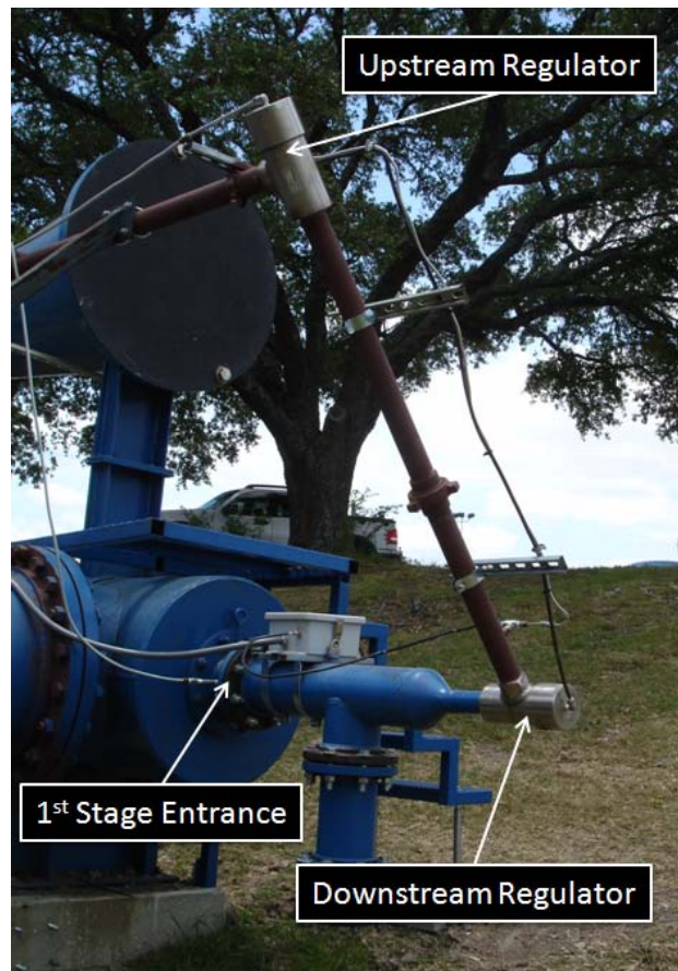
Figure F-6: Ejector 1 st Stage Air Supply Line
