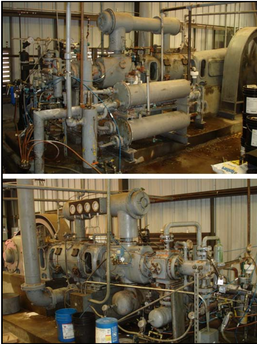
Figure 7: Chicago Pneumatic Compressors
