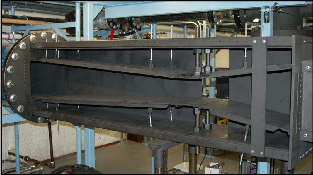
Figure F-101: Installed Diffuser
