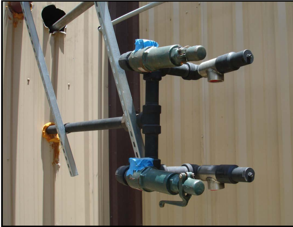
Figure 33: Heater Room Safety Relief Valves
