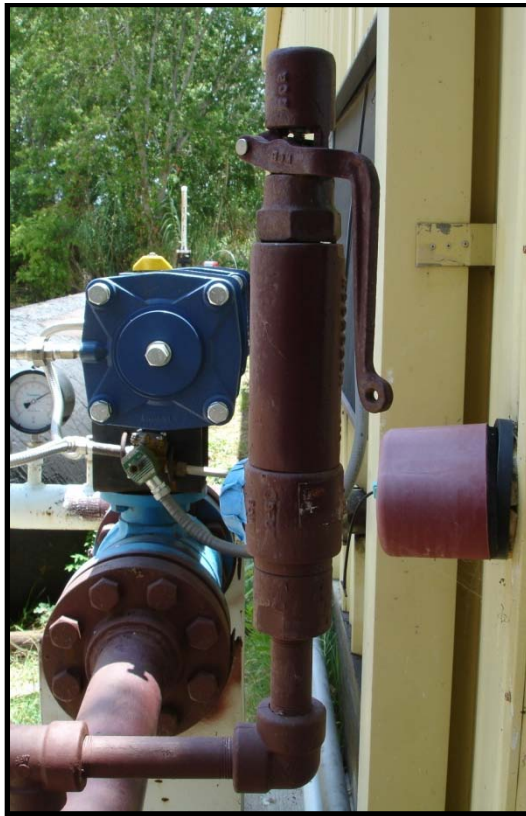
Figure 25: High Pressure Hydroseal Safety Relief Valve
