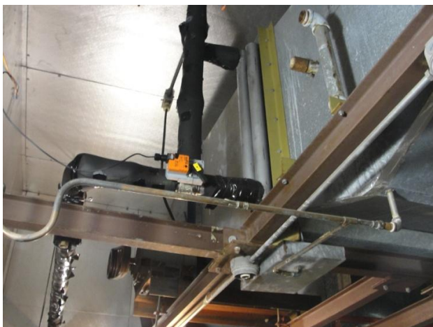
Figure 2. Photograph of the current cooling coil piping.
