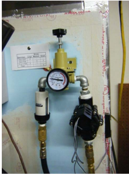
FIG. 5-26. Pneumatic System Controls
