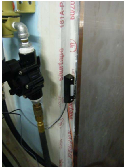
FIG. 5-25. Pneumatic Cylinder Air Injection Engagement Switch
